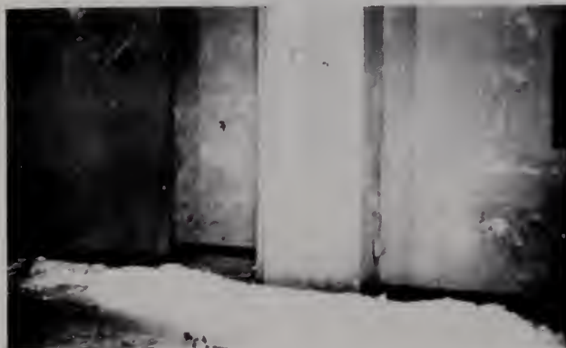
Wet plaster from ceiling covers table
